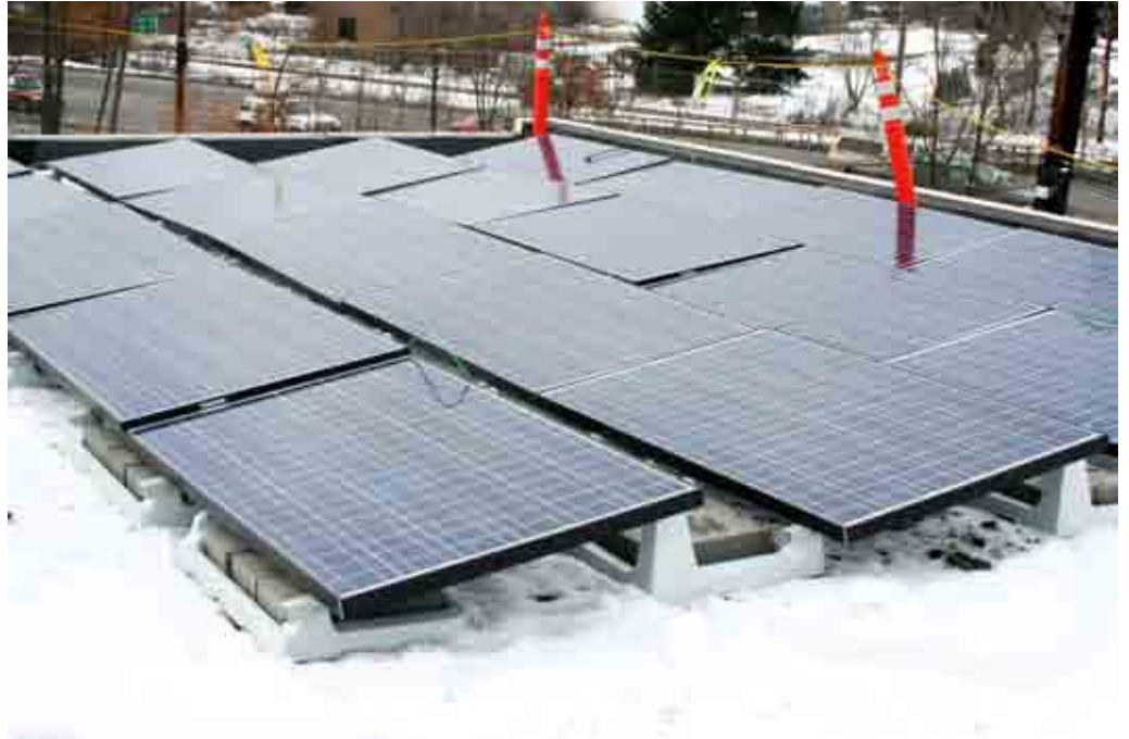
Solar panels were added to the roof of the CCE-Tompkins Education Center in January 2013. Cost savings are estimated to total $4000 per year.
