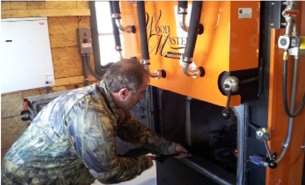
Firing up the new pellet boiler at Schaefer's Gardens Greenhouse, one of the 2016 demonstration sites in this project
