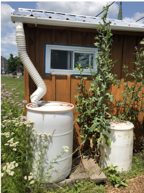
Rainwater system at Hornell YMCA
