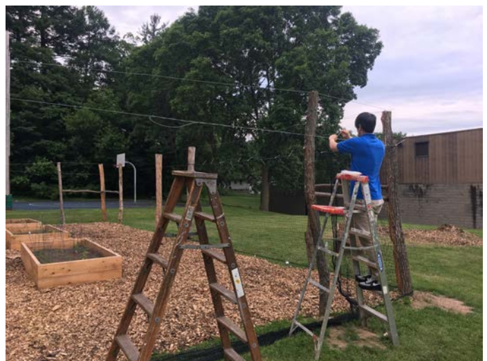
Brandon Wakeman works on installing a deer fence at Booker T. Washington Community Garden in Auburn
