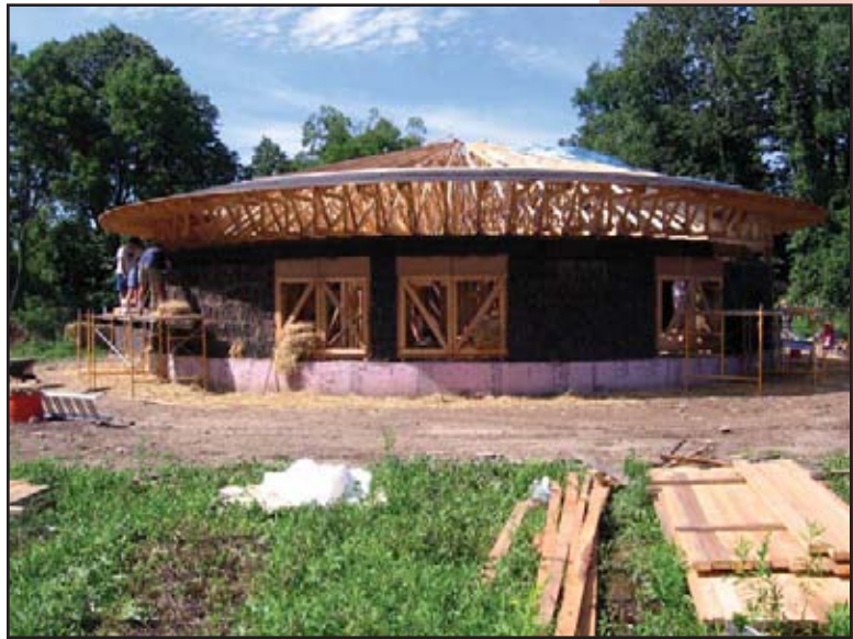
This straw-bale home in Freeville was under construction during the 2007 Tour, allowing visitors a view of many construction details.
