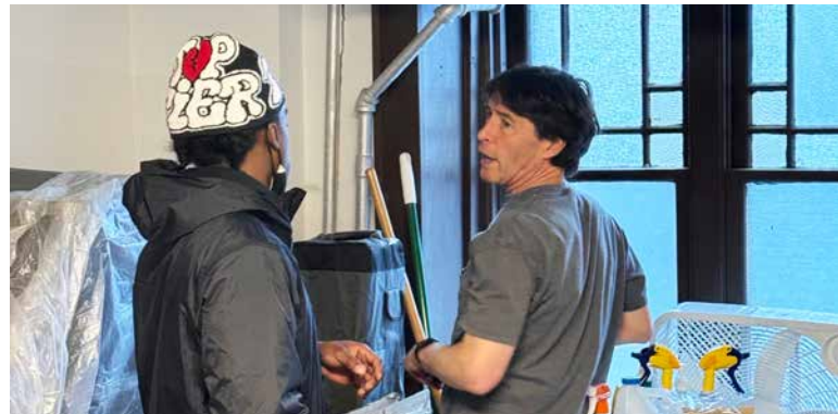
Cozy Basements project work at AME Zion Church, a historic building that has hosted Frederick Douglass, Harriett Tubman, and other distinguished Black leaders.
